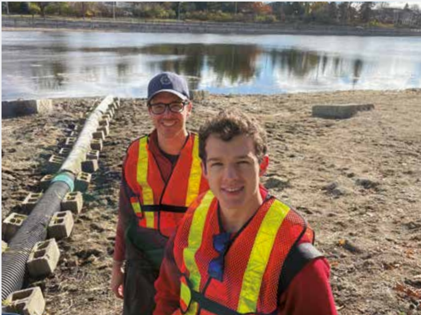
Carleton University Professor Cole Van De Ven, at left, and environmental engineering student Chris Rouse install sensors in the Rideau Canal in Ottawa in late 2022. Photo: Yeowon Kim
